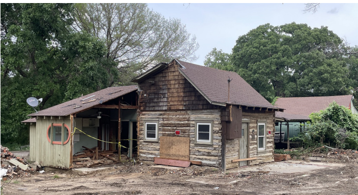
May 2024: Twentieth-century additions are cut away from the house before the move.
